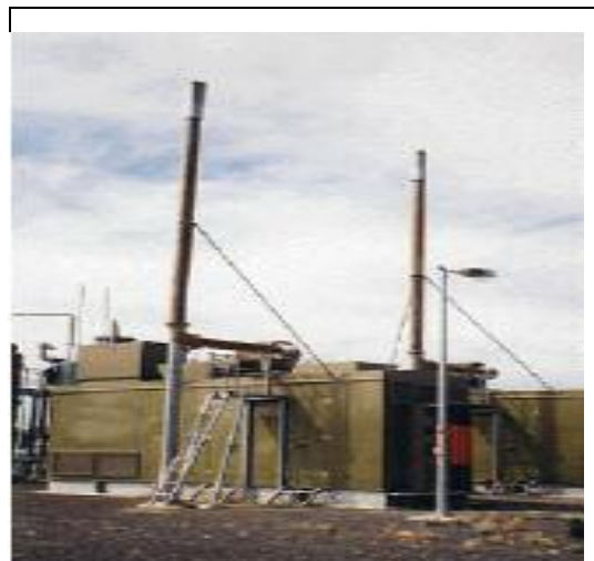
600 kW generating plant fuelled by biogas
